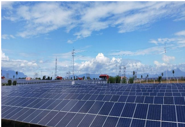
Solar Plant – Jew ISCM
