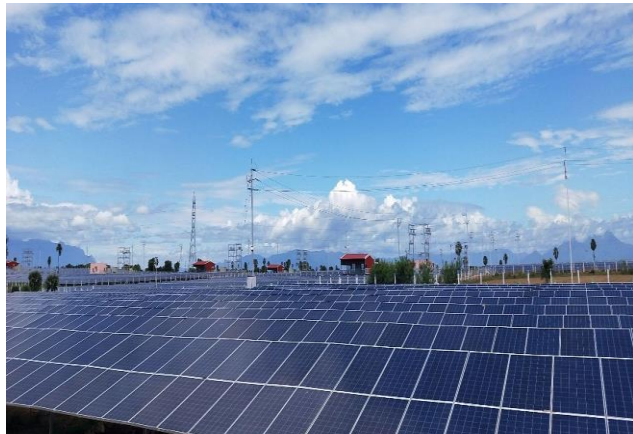
Solar Plant – Jew ISCM
