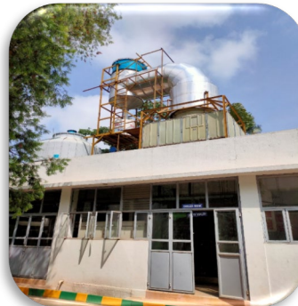
Evaporation water recovery Cooling towers in Jewellery
