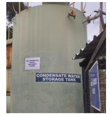
Condensated water recovery
